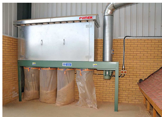
Fig. 2.18: Example of Dust Extraction System
